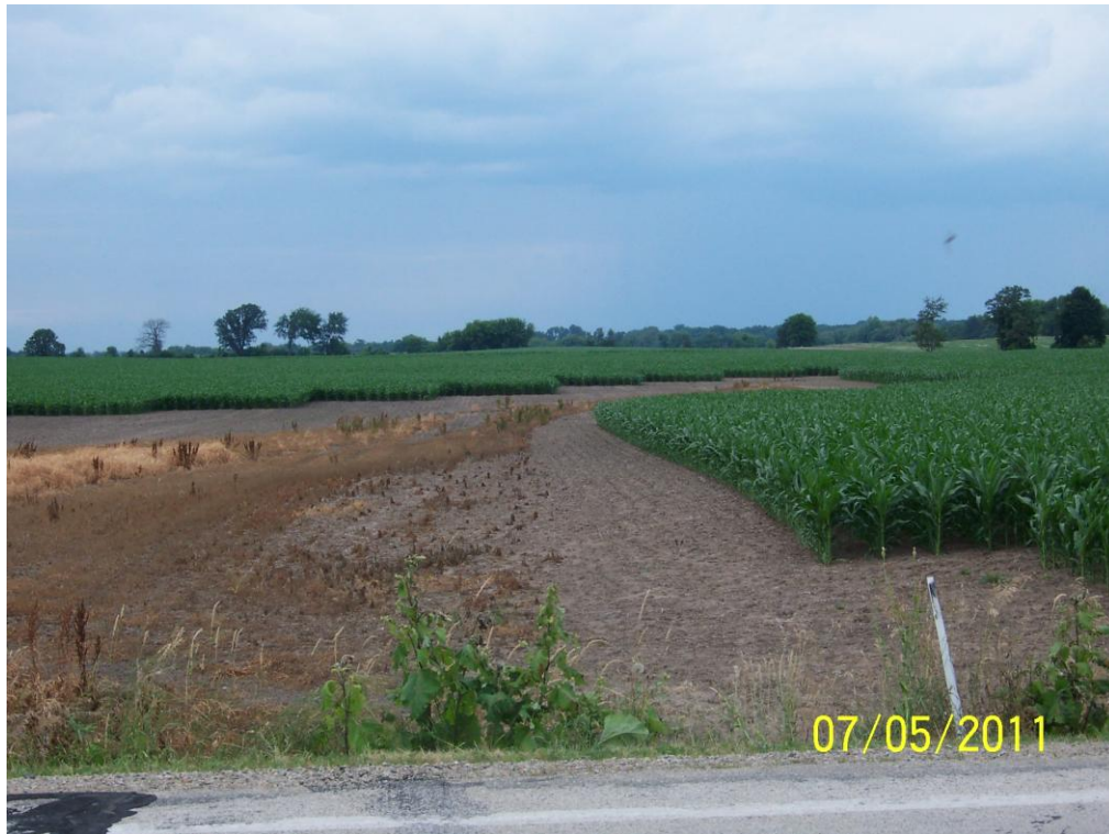
Figure 8. Looking north from culvert at Highway B showing the drainage way with an herbicide-treated zone near the centerline of the drainage way and bare, exposed soil with no cover vegetation on either side of the centerline.
